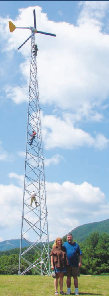
Doug and Mary McCallum at the base of their turbine as workers finish it.
