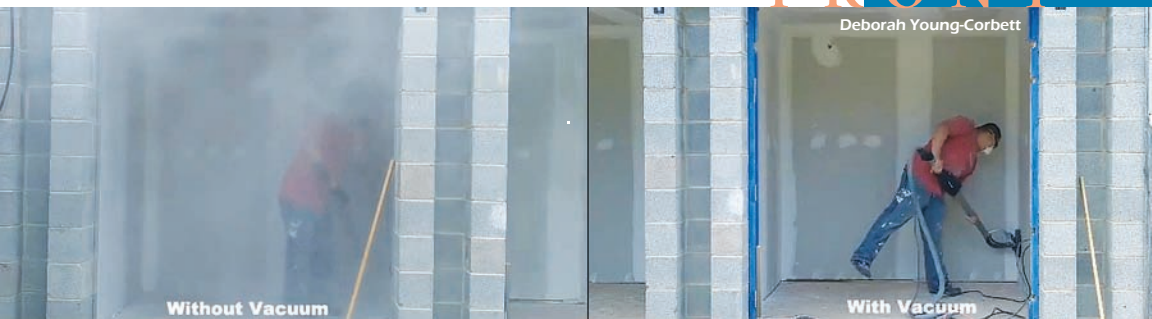
Left: Worker sanding a wall. Note the dust in the air. Right: Worker using a sander designed by Young-Corbett and her team. The tool's built-in vacuum removes 99 percent of the dust.
